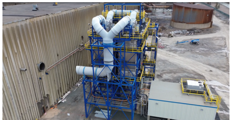
Wet Electrostatic Precipitator ducts disconnected to create separation between Acid Plant and equipment
