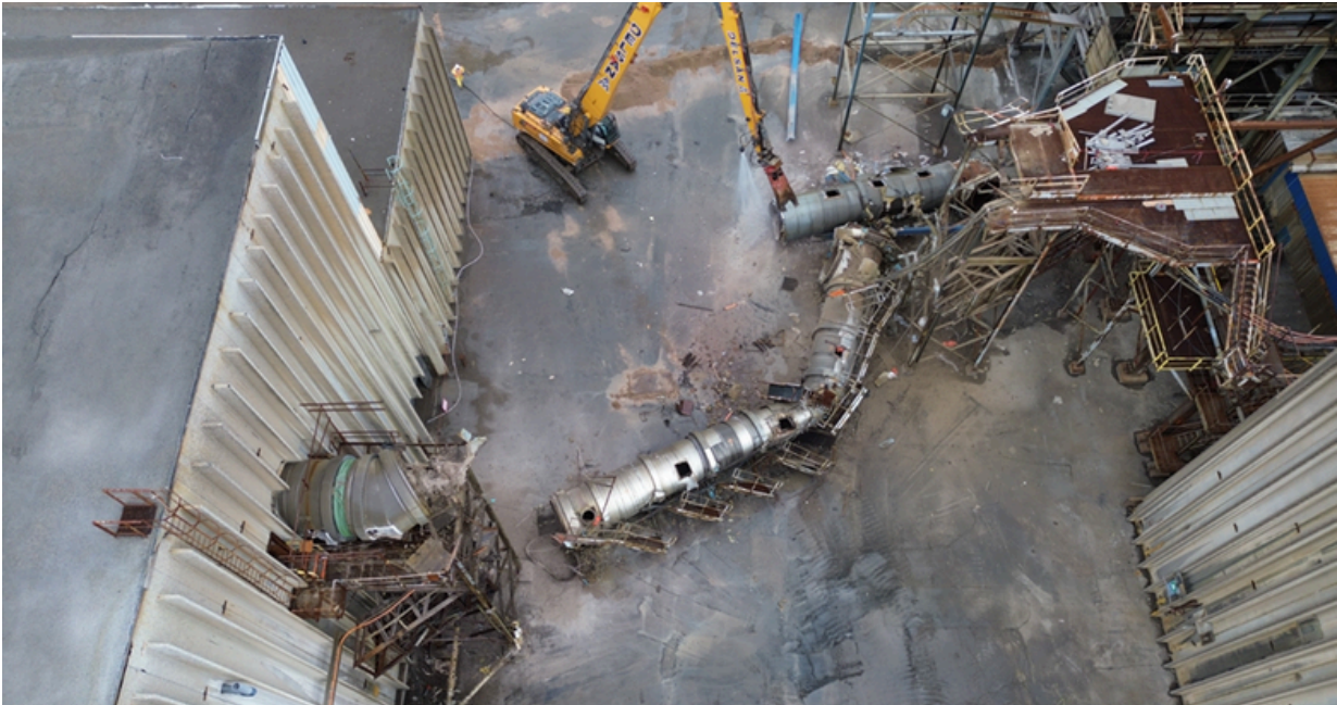
Hot Gas Precipitator outlet duct on the ground
