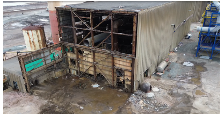
Contact Section and lower roof area at west end of Acid Plant demolished
